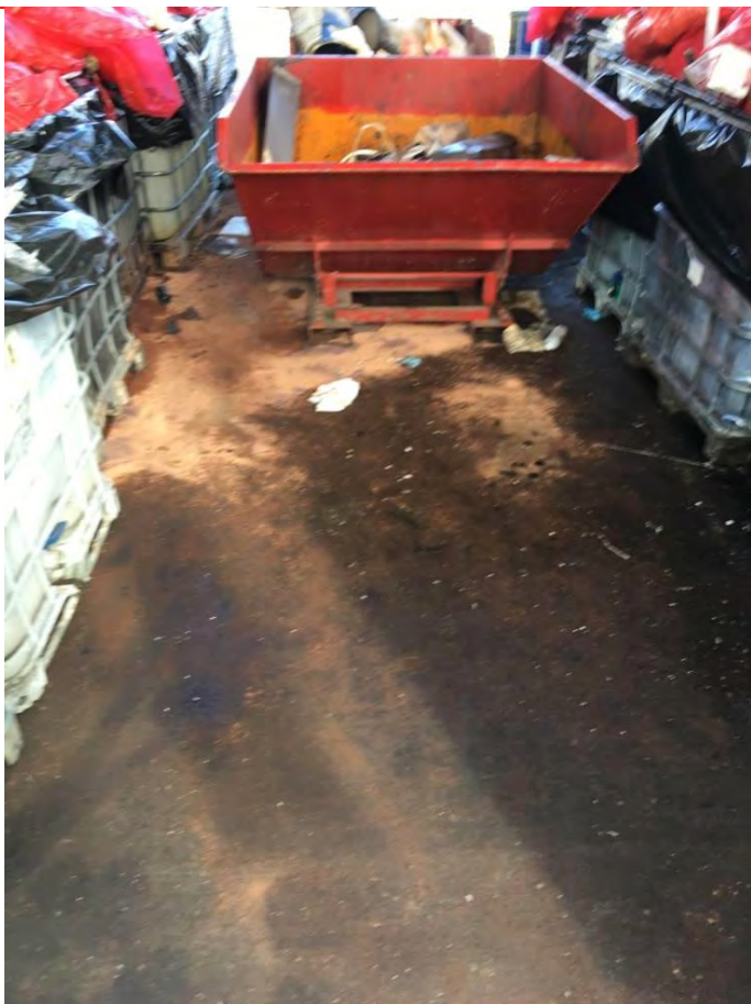
Plate 39: Staining across the hardstand of the Hazardous Waste Storage Area in the centre of the Assessment Site (facing north)
